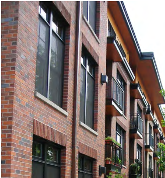
Fig. B.5.S13: Recessed windows provide a sense of depth and shadowing on the residential facade.
