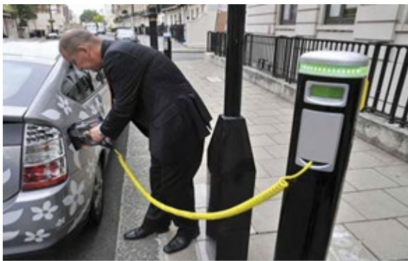
Single Electric Vehicle Charging Station on Street
