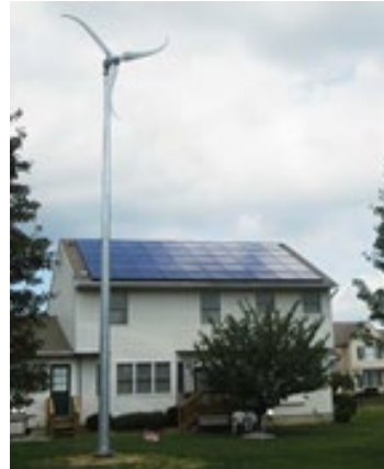
Small-scale, blade-type wind turbine mounted on a pole.
