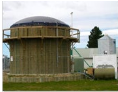
Biogas/Methane Production Facility
